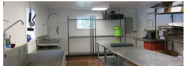
This wash area has stainless steel spray table and triple-basin sinks as well as dry-pack tables. Shelving conveniently houses waxed boxes. Lights are covered with shatter proof plastic. The painted concrete floor is easy to clean and contains a floor drain. Mats make standing for long periods easier on workers. The handwashing sink is located to the rear. Tianna DuPont, Penn State Extension
