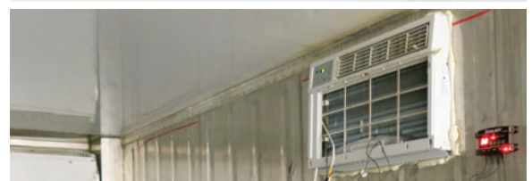
CoolBot control system and air conditioner for a small cold room. Roots to River Farm
