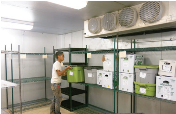
Room cooler. Andrew Puglia, Hillside Farm
