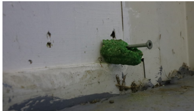
Rodent bait near a doorway close to the floor.
