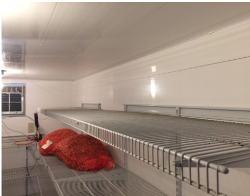
Smooth, clean and shiny, this CoolBot™ cooler used TrussCore™ twinwall PVC as a finish surface.
