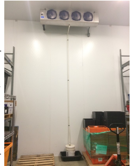
This cooler has no floor drains. Instead the evaporator drain is plumbed to a bucket that is emptied according to an SOP.
