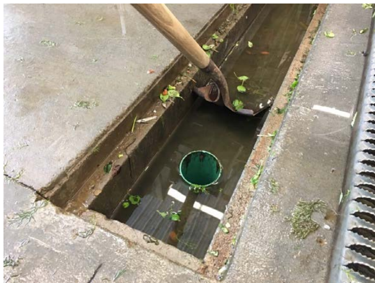
This trench drain was designed with a wide opening to make shoveling sediment easier. The green standpipe raises the top level of the water during use allowing sediment to settle out. The removable covering grate is shown at left.
