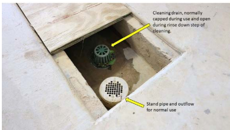
Outlet details of a trench drain showing the standpipe and cleanout drain.
